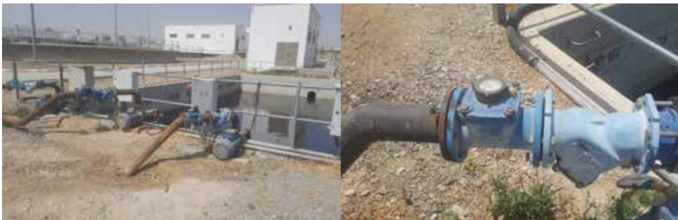
IMAGE 5.3 Effluent storage and irrigation tank and the effluent pumps and the flow meters at Jericho WWTP. Photos: I Abu Seiba.
